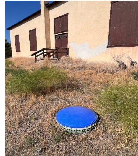
Septic system cover on the northeastern corner of the building on the Subject Property
