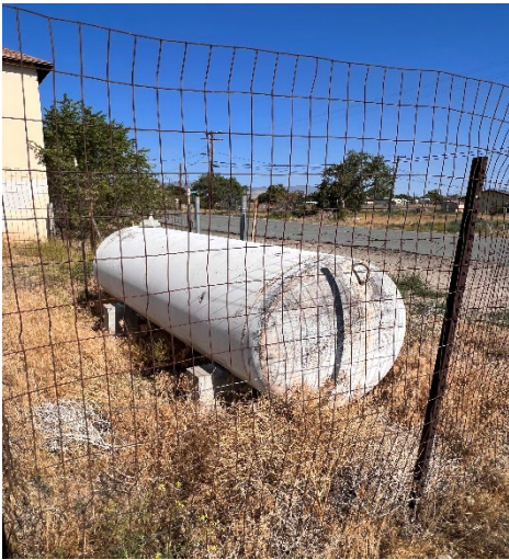
Propane tank on the Subject Property
