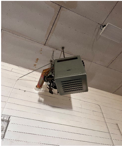
Space heater located inside the gymnasium
