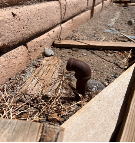
Potential heating oil tank piping on southern portion of the Property
