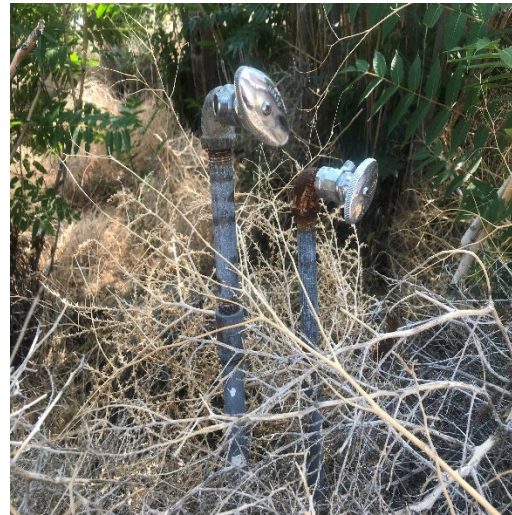
Potential heating oil tank valve on the northwestern portion of the Property
