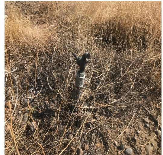
Potential heating oil tank valve northern portion of Property
