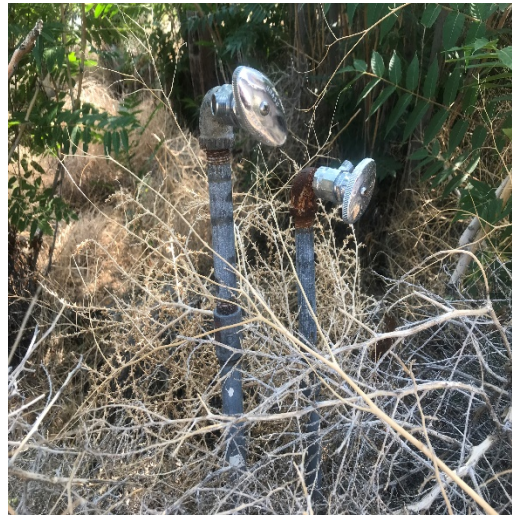
Potential heating oil tank valve on the northwestern portion of the Property
